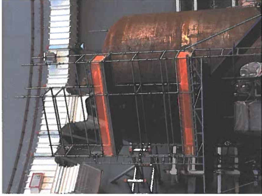
Unit 2 Installed Steam Generator with Protective Oxidation
