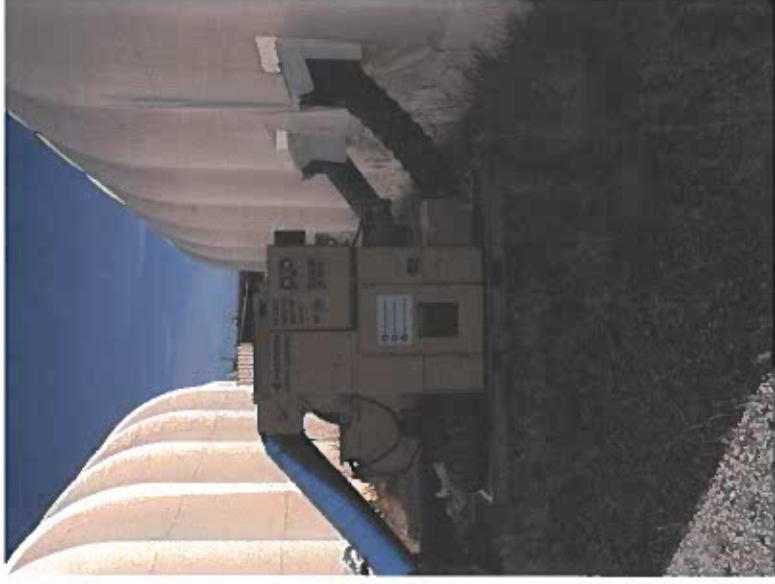
Dehumidifiers in place for Diesel Generator tent
