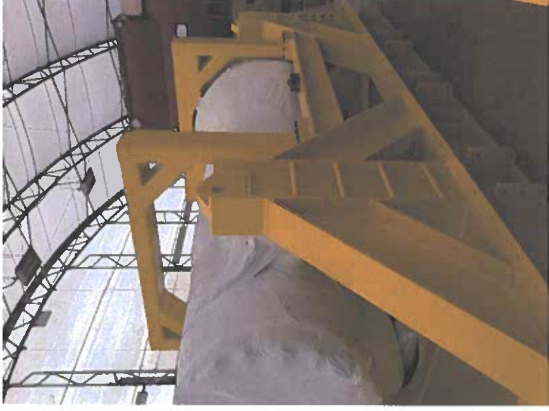
Reactor Coolant Pump in storage
