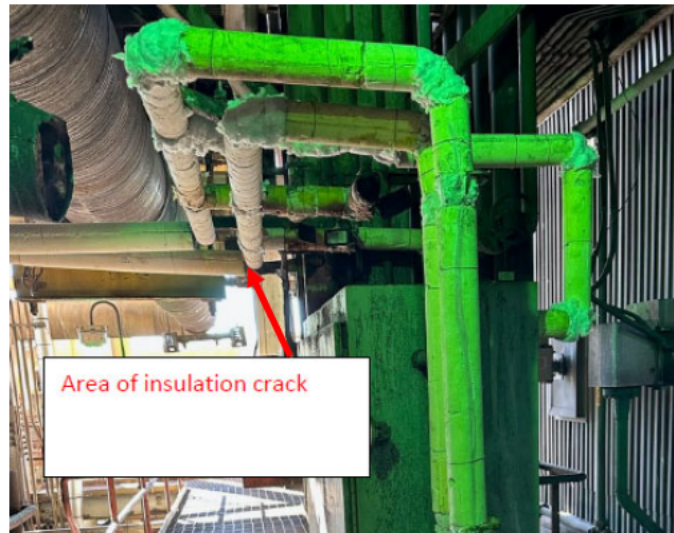
Figure 3-11: Cracked Insulation on Sensing Lines Discovered at Roxboro Unit 3 liv
